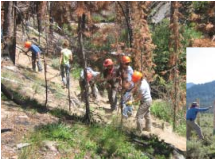
High-school-age girls and boys from Landmark Volunteers construct a trail along Pigtail Creek in the White Cloud Mountains. The area was burned last year by a 40,000-acre wildfire and erosion this spring blew out a section of the original trail that leads to Warm Springs Meadow. The Sawtooth Society has sponsored Landmark Volunteer work parties to the Sawtooth National Recreation Area since 2000.
